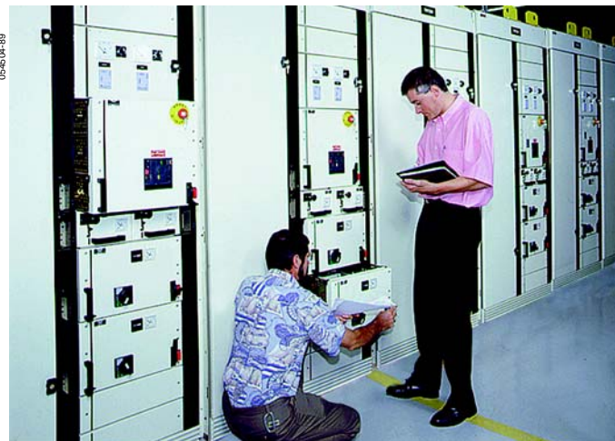
Motor Control Centre (MCC).
